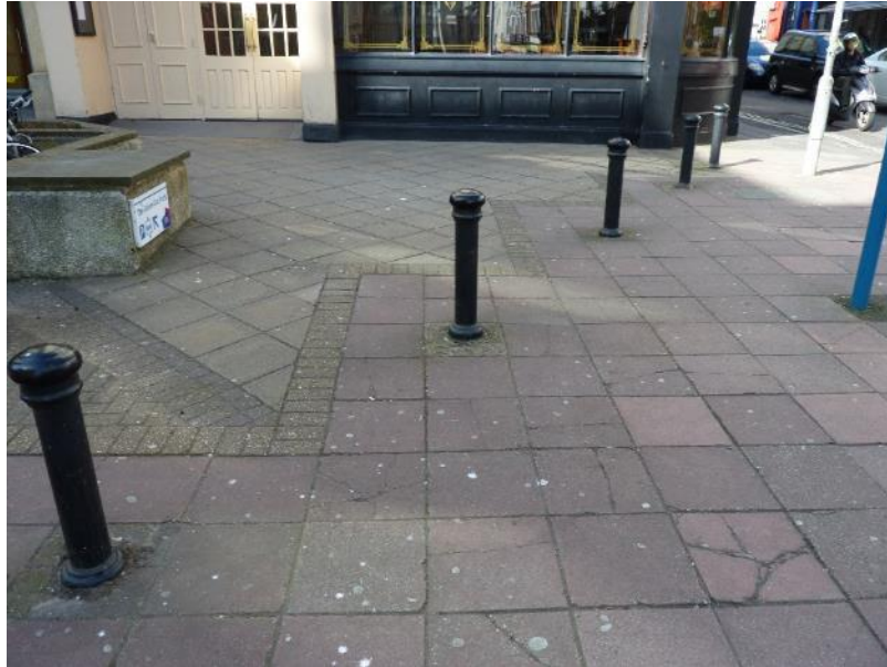
Bartholomew Square: incoherent street surfaces poorly maintained
